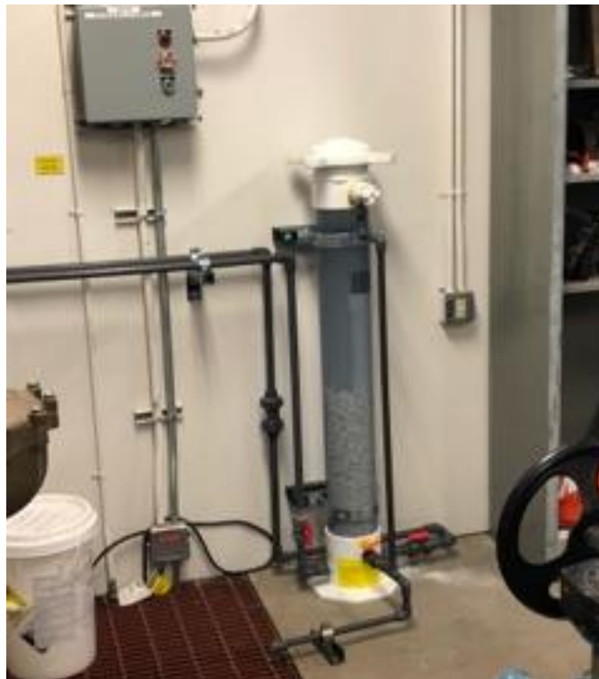
Photograph - NPDES-03A113-18-006 TA-53-952 Cooling Tower Brominator Located in TA-53-950
