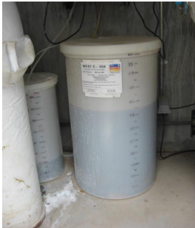
Photograph - NPDES-03A113-18-010 TA-53-293 Chemical Treatment Feed Tanks Located in TA-53-1038 [Inactive but Available for Use]
