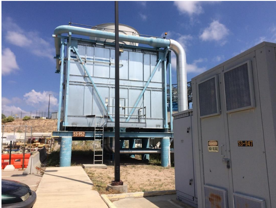
Photograph - NPDES-03A113-18-005 TA-53-952 Cooling Tower
